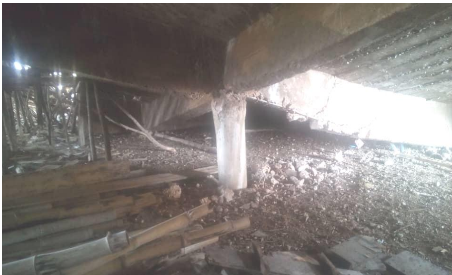
Plate 2: Inner Portion of the Collapsed Building showing a sunken column
